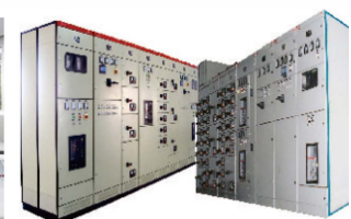
Series of electrical controlled equipment area
